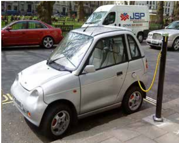
Electric vehicle charging point.
