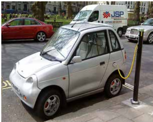
Electric vehicle charging point.
